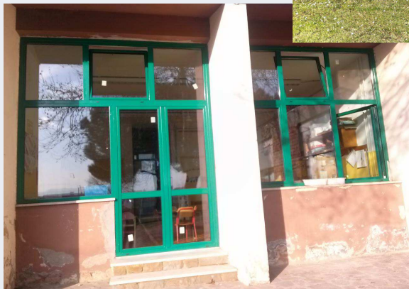
Primary school Meoni in Prato: noise abatement windows
